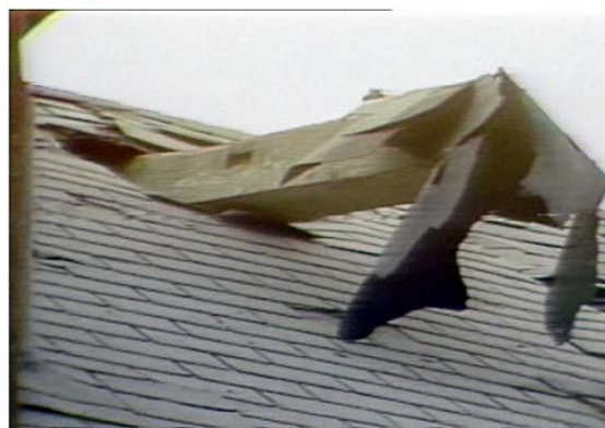
This video still shows a beam that penetrated the roof of a residence during the tornado. Video still courtesy of WBNS-TV Film Archives Department
