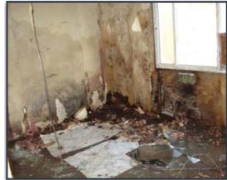
Interior photo of the Little Avenue home prior to demolition. Exterior walls and flooring shows water stains, mold and mildew.
