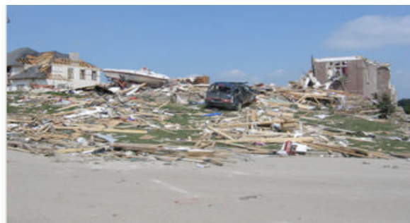
An example of F3 damage. Here, the roof and some inner walls of this brick building have been demolished. While taking shelter in a basement , cellar , or inner room improves your odds of surviving a tornado drastically, occasionally even this is not enough. F3 and stronger tornadoes only account for about 6% of all tornadoes in the United States, and yet since 1980 they have accounted for more than 75% of tornado-related deaths.
