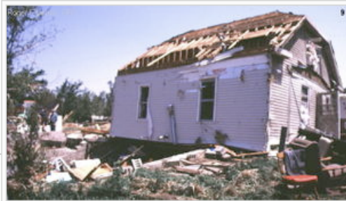
An example of F1 damage. F1 tornadoes cause major damage to mobile homes and automobiles, and can cause minor structural damage to well-constructed homes. This particular mobile home appears to be a double-wide, and it was still moved off its foundations , with its roof badly damaged. A mobile home or car is a very poor shelter, even during severe thunderstorms which do not contain a tornado.
